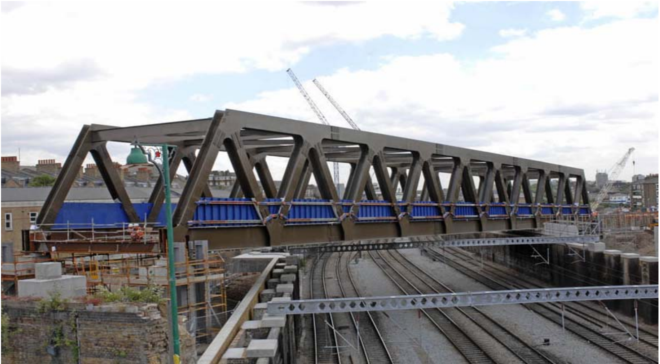
GE19 in position across Network Rail tracks outside Liverpool Street Station shortly after its launch
