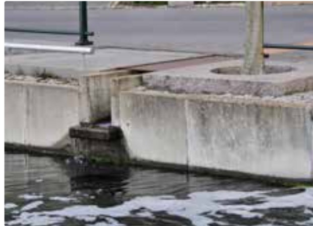
5. Discharge to watercourse
