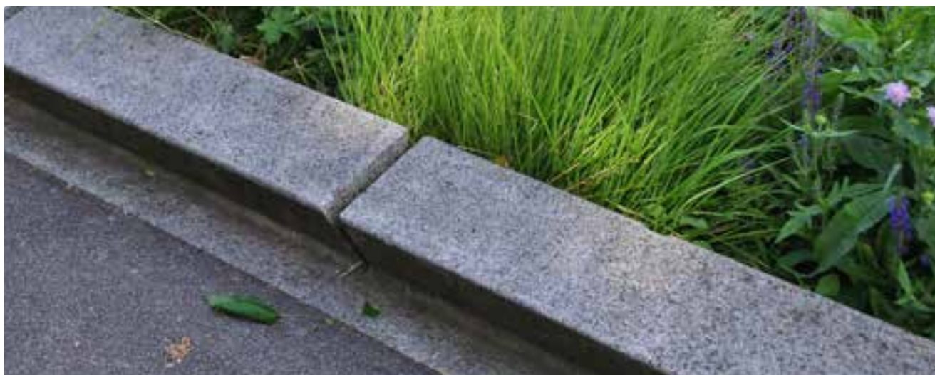
Broken kerb detail for bioretention
