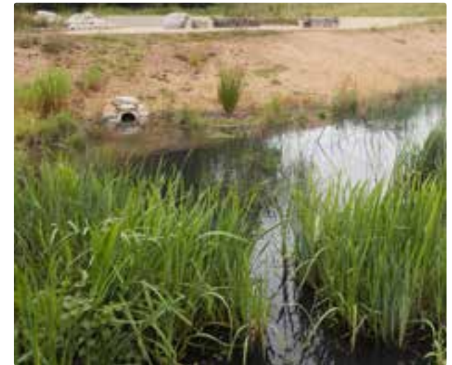
Outlet into wetland area
