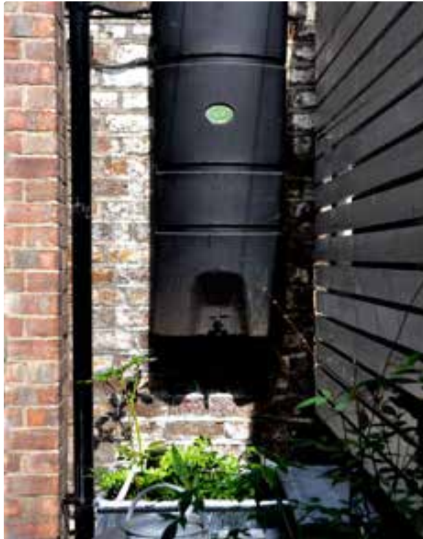
1. Disconnected downpipe to water butt
