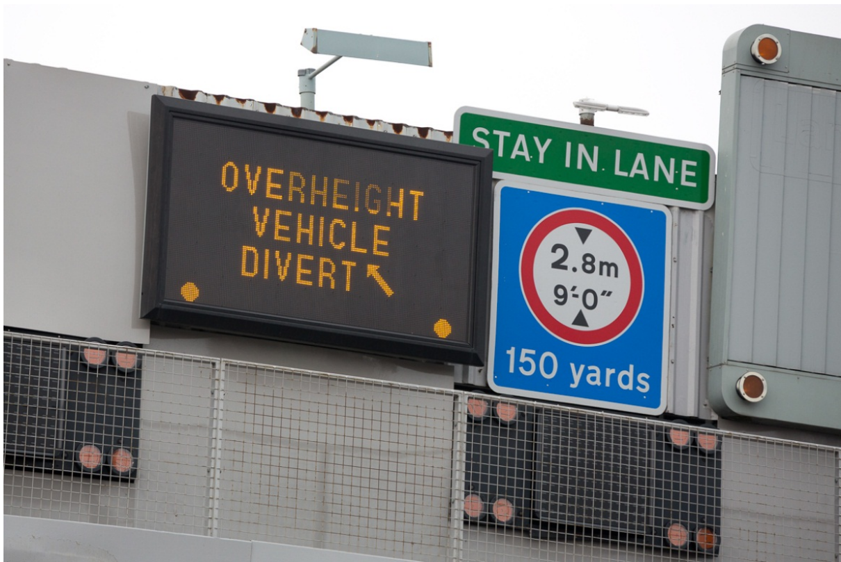
Figure 20 : Overheight vehicle detection sign
