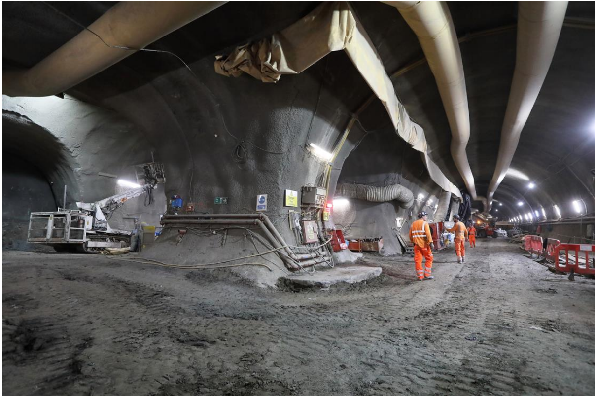
Figure 5: Tunnelling the new southbound Northern line and cross passageways (excavated 1000m of a total of 1,300m of tunnels).
