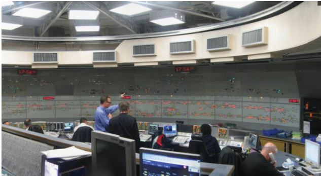
Figure 1 – Earls Court Control Centre (left); Griffin Rooms (right)
