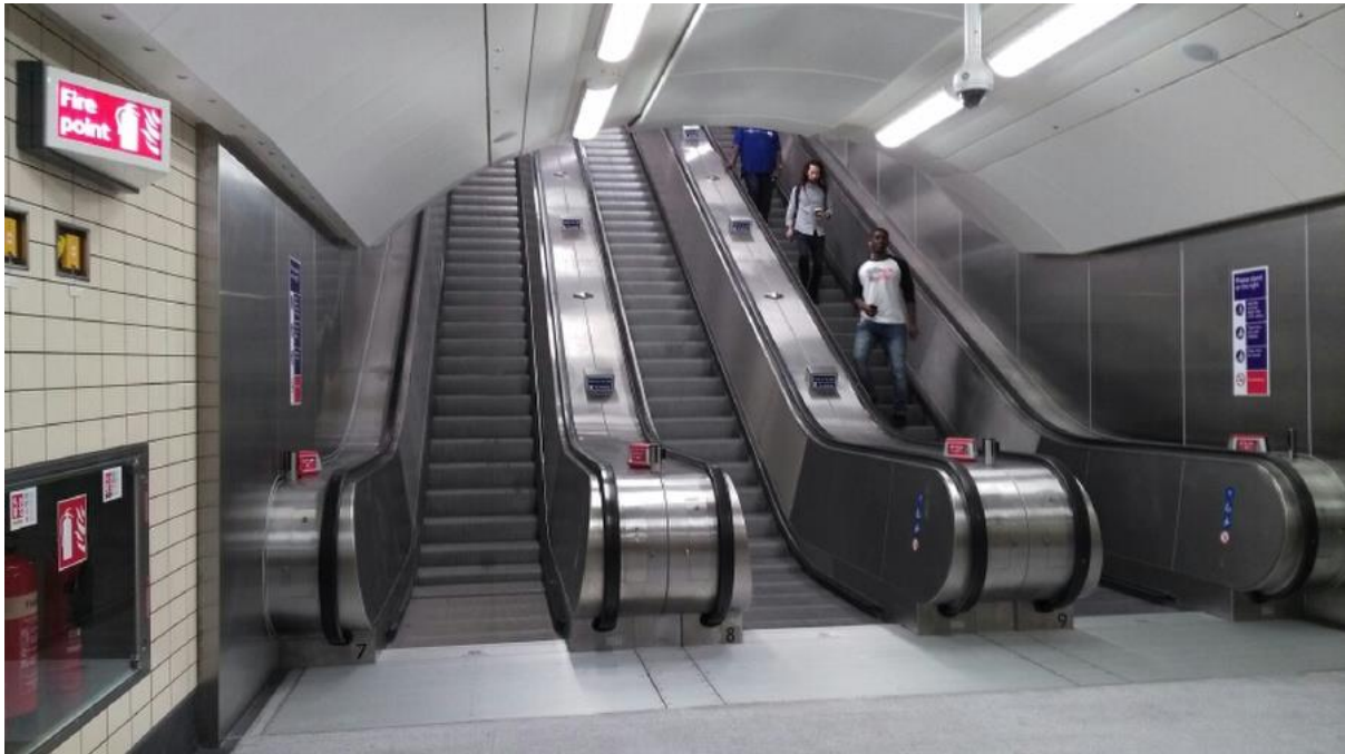
Figure 1: New escalators installed as part of VSU.
