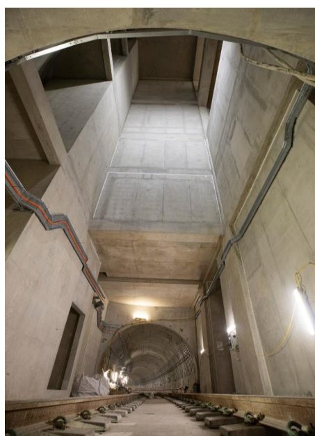
Fig.1 View from the bottom of the shaft showing internal rooms, cabling and the tunnel path
