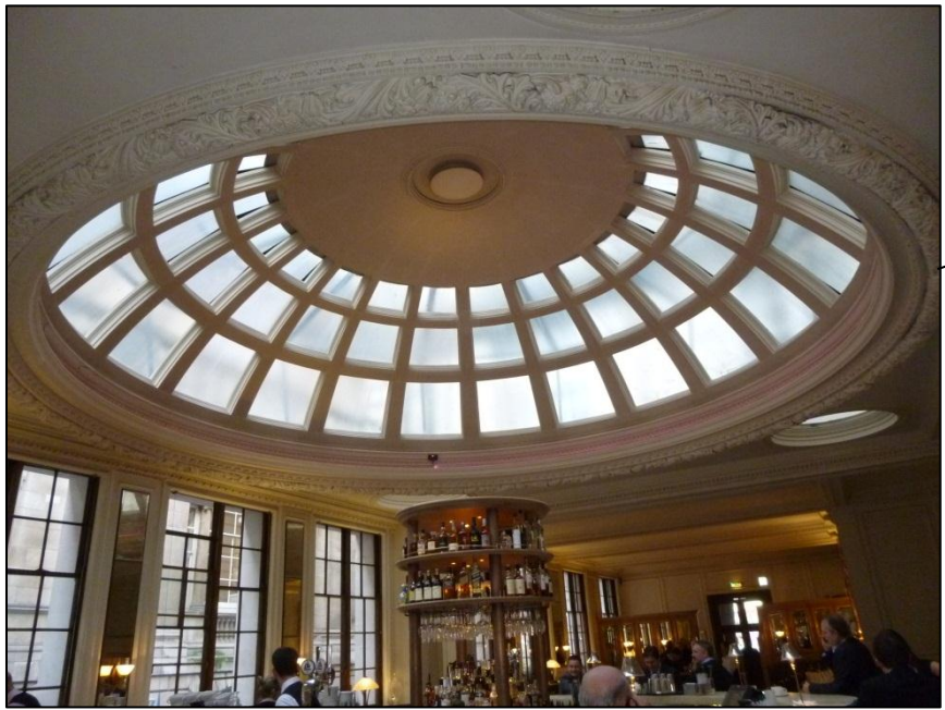
Large dome in restaurant with plaster enrichments to rim, in poor condition
