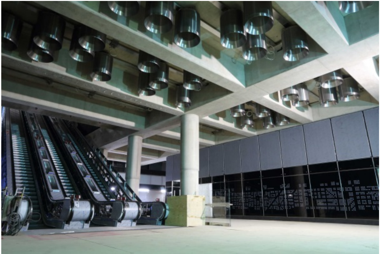
Tottenham Court Road station
