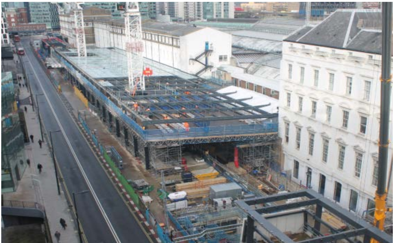
Paddington Station – installation of the station canopy incorporating ‘A Cloud Index’ by Spencer Finch, part of the Crossrail Art Programme
