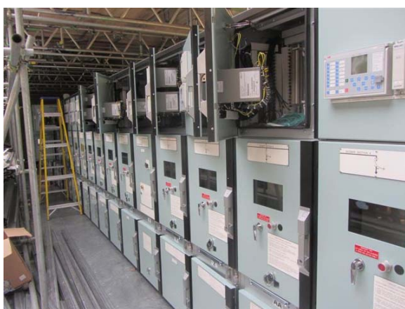
New 11,000 volt switchgear during pre-commissioning phase at Ravenscourt Park
