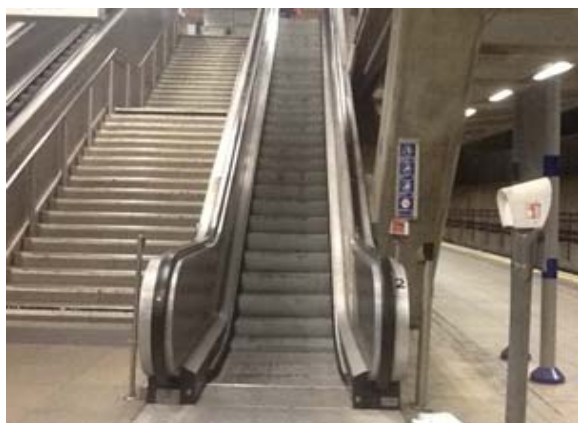
Escalators at Canning Town station
