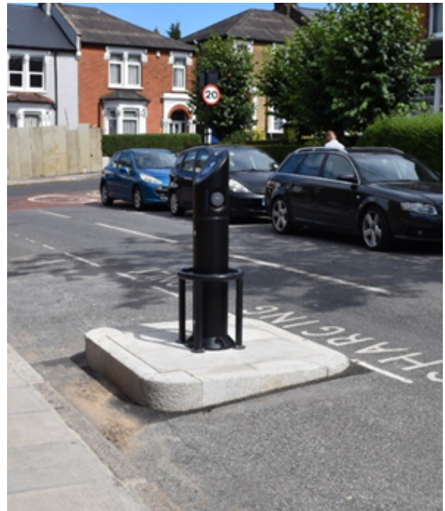
Figure 7: An on-street charge point installed on a build out in the road in Haringey, London
