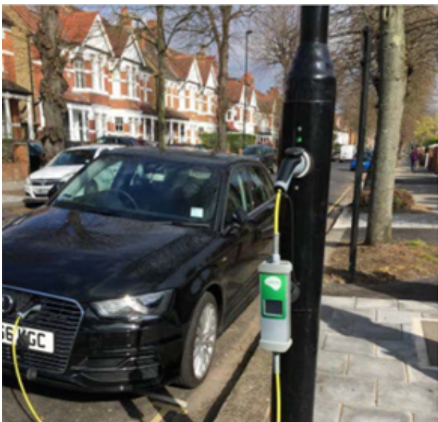
Figure 6: Lamp column charge point in London
