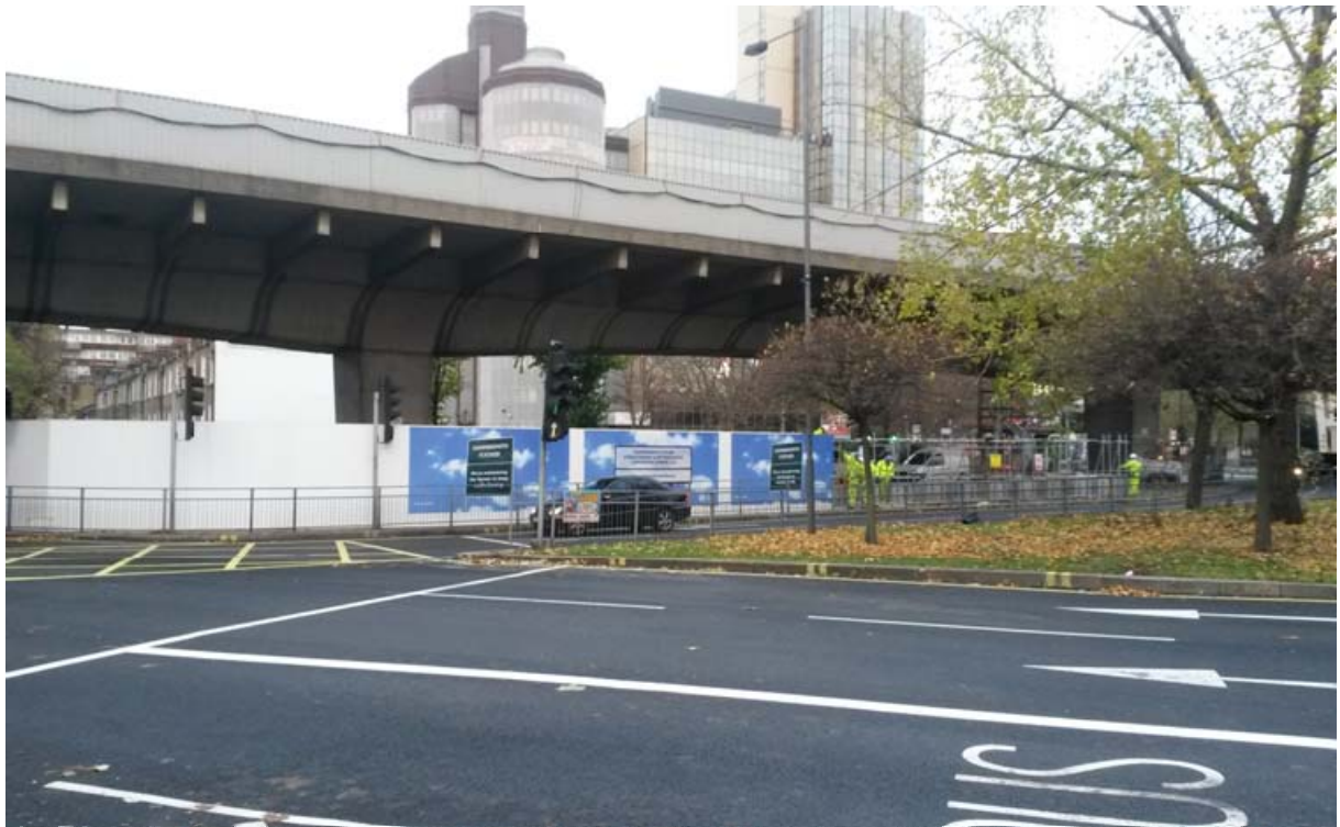
Site establishment with erection of hoarding and scaffolding to access the flyover from underneath
