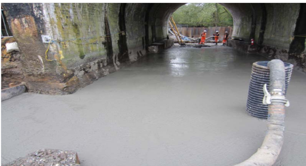
Concrete pour complete and settling prior to diverting the river to flow as normal
