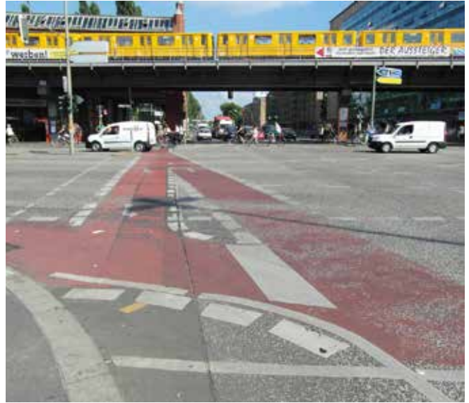
Rather worn markings for ahead and two-stage left turns
