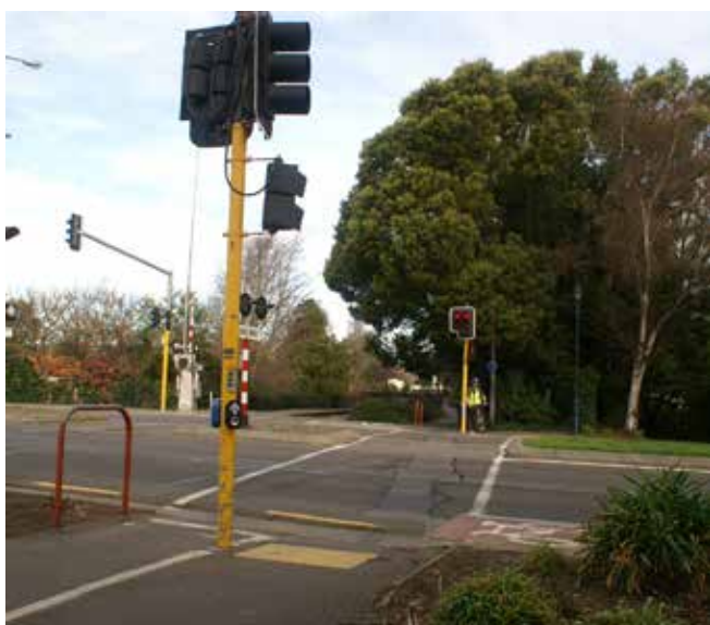
Advanced loop detection creates green wave on cycle path
