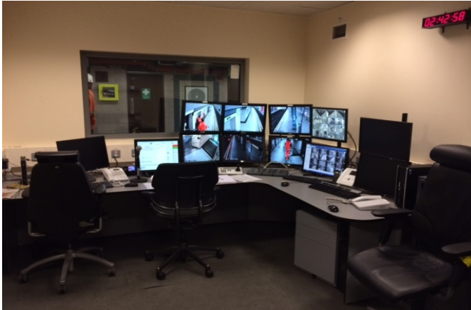
New Control room delivered at Moorgate
