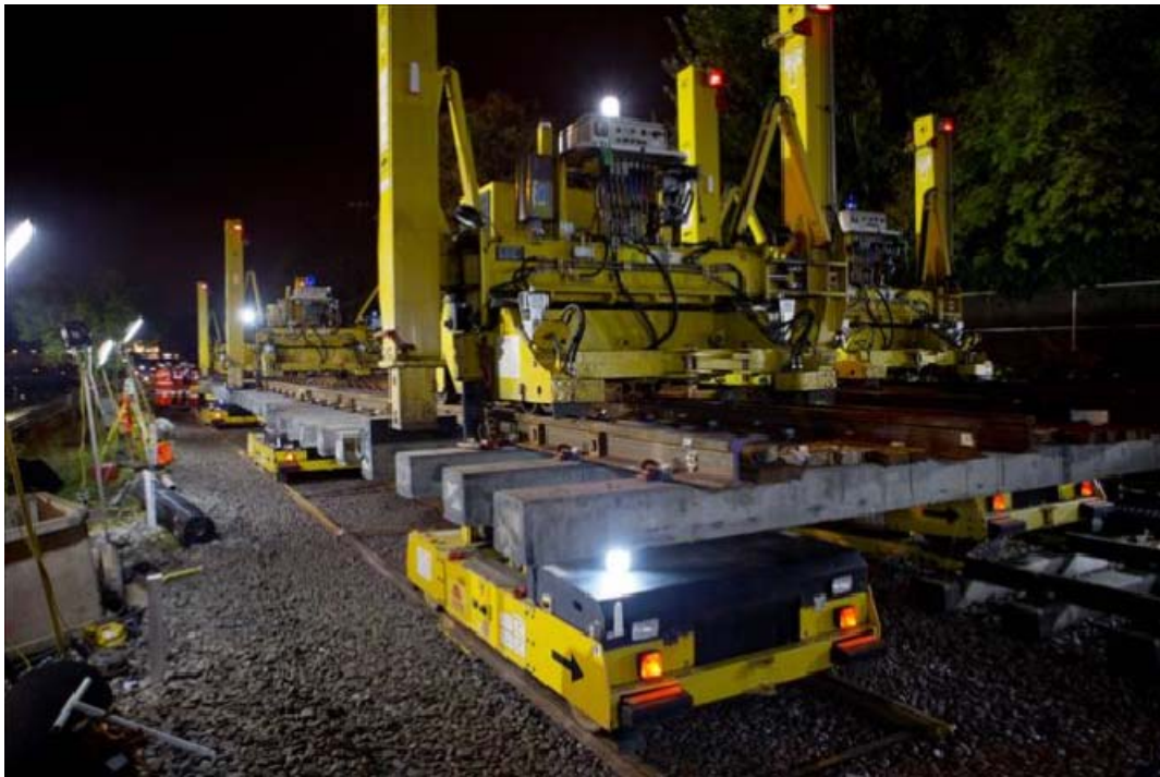
The remodelling and installation of a critical section of the network at Acton Town
