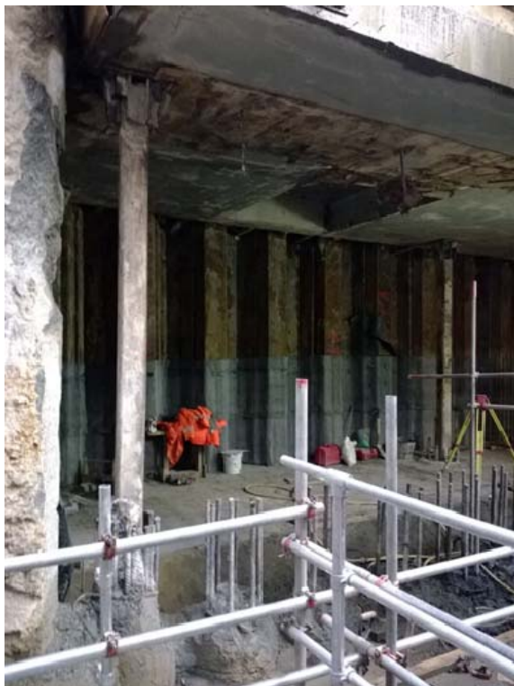
Substation piling broken down
