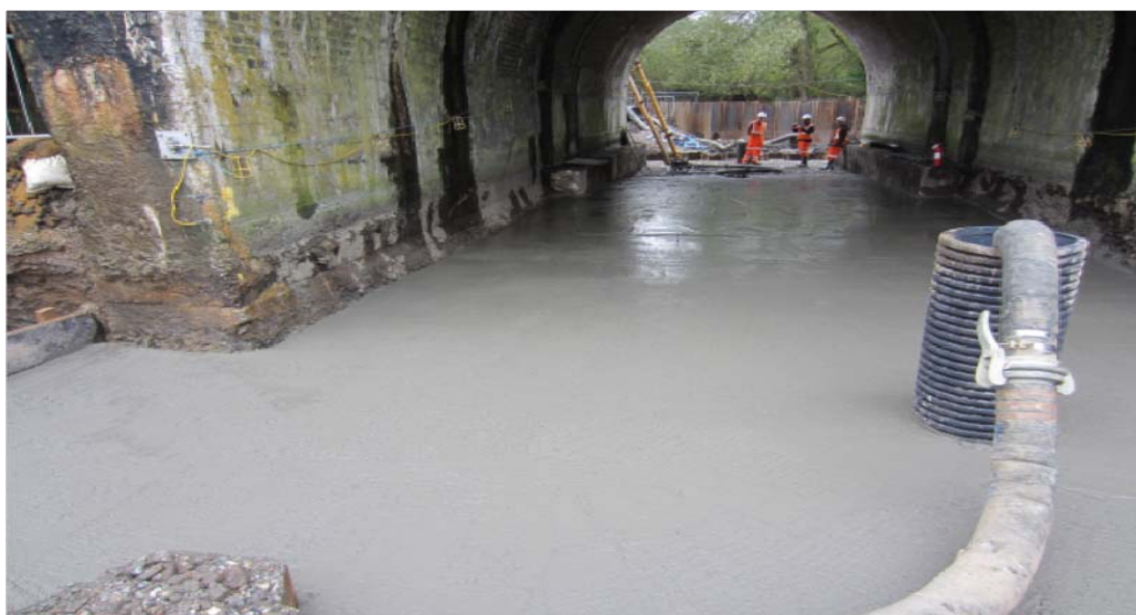
Concrete pour complete and settling prior to rediverting the river to flow as normal
