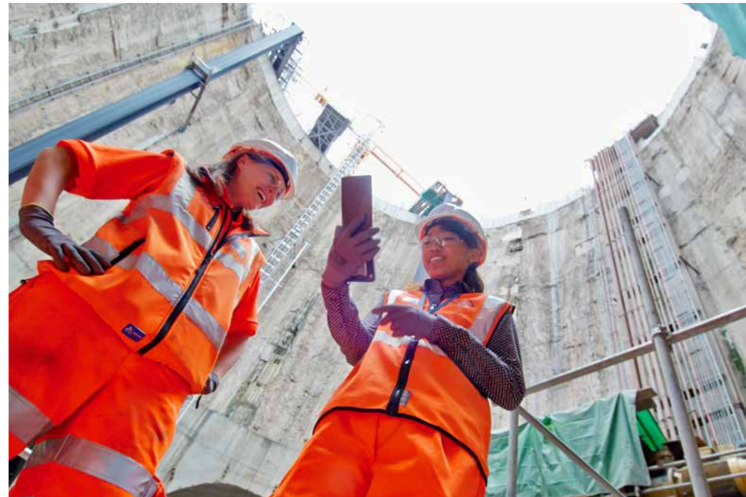
Women in engineering Members of our graduate scheme at work in new Crossrail tunnels
