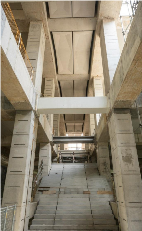
Photo 2: The installation of pre-cast concrete stairs from ticket hall to platform level has been completed.
