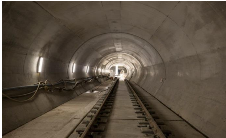
Photo 4: Track has now been installed in the tunnel sections between the two new stations.
