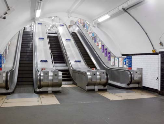
Completed escalators at Chancery Lane station
