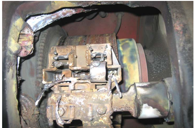
Existing motor as a result of a flashover
