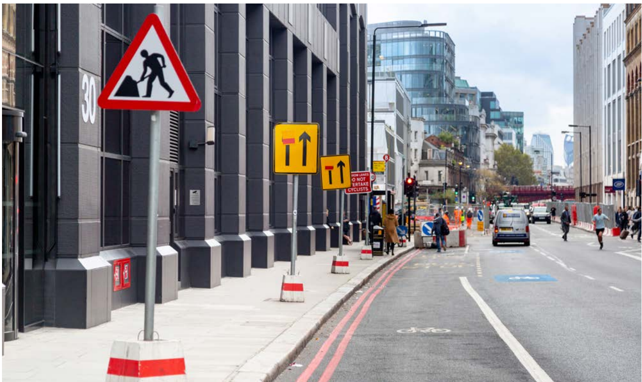
Alternative sign mounting reduces trip hazard and sign maintenance
