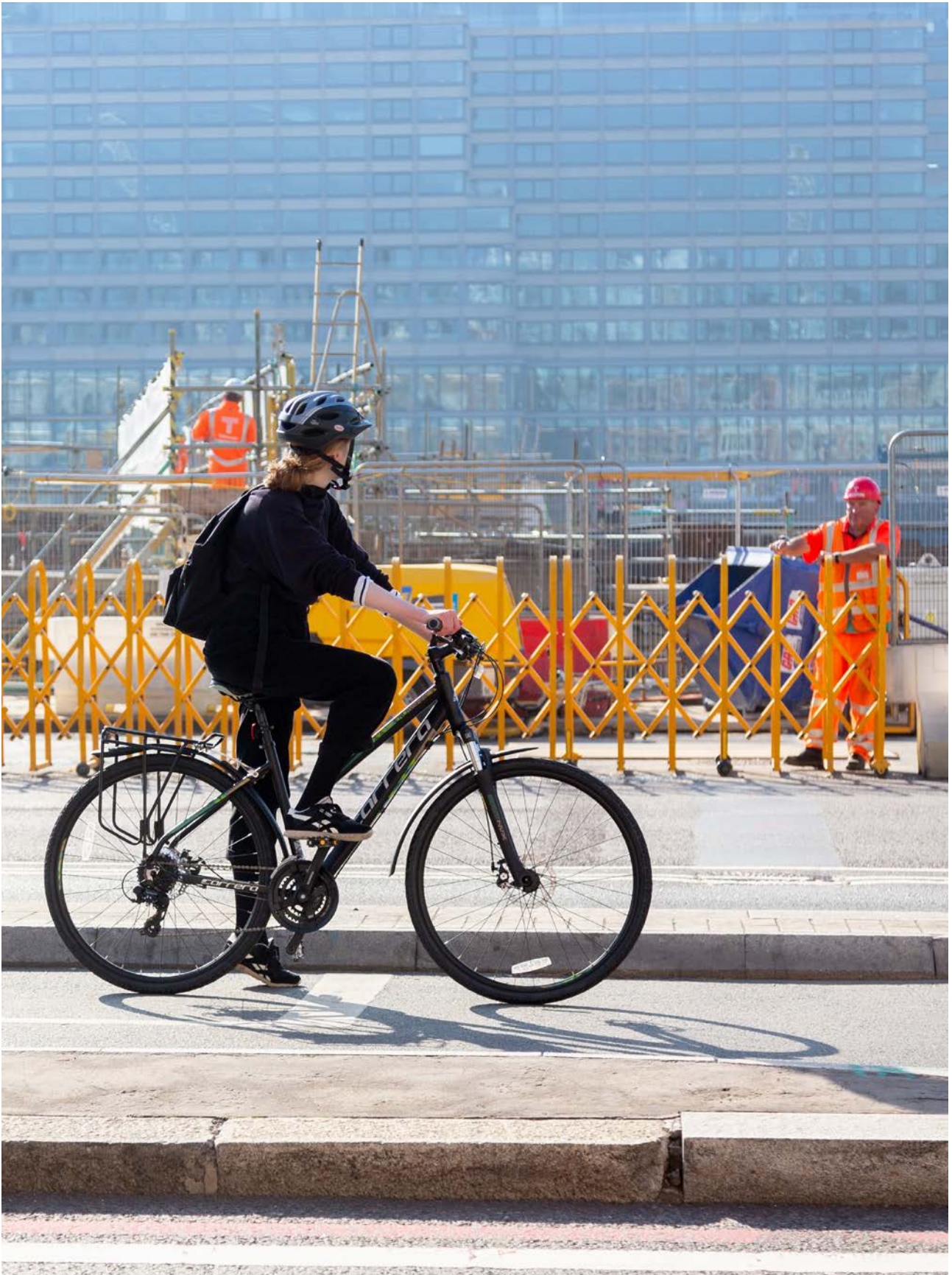
Retractable barrier system marshalled to allow site access
