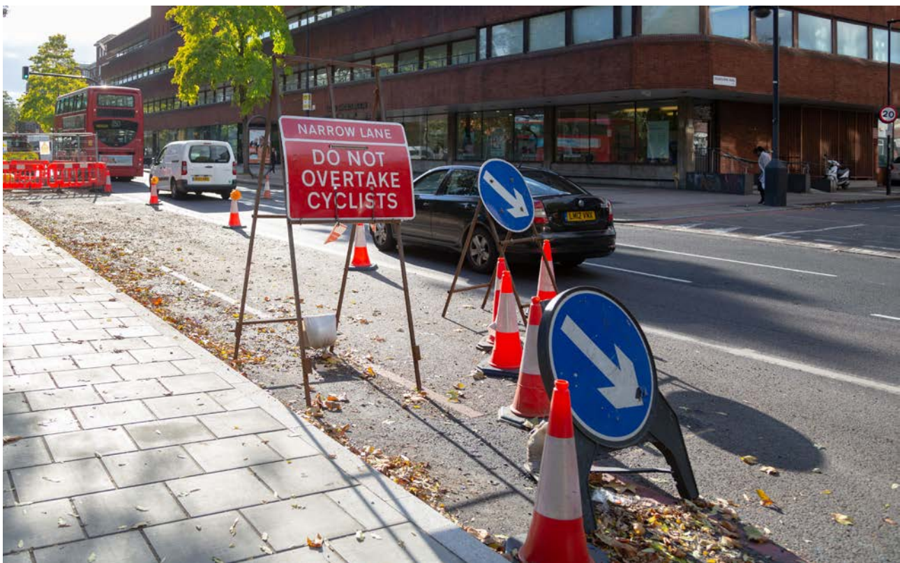
Correct warning sign
