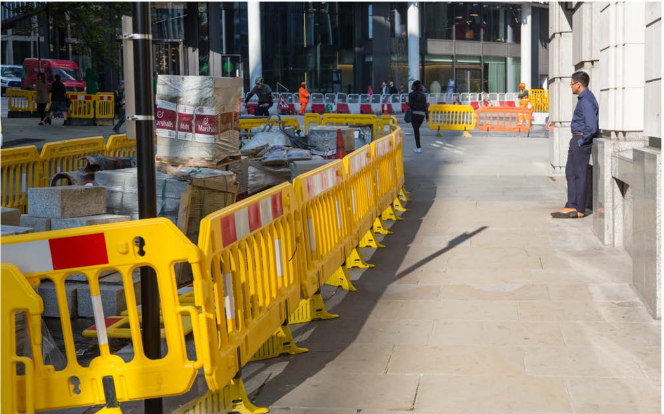
Good practice: tidy, correctly assembled and well-maintained barrier
