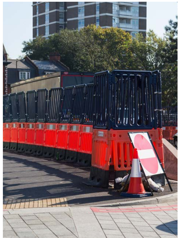
Straight and tidy barriers maximise safety and give a good impression on site
