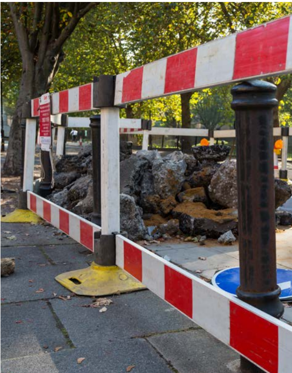
Barrier systems with large gaps can easily be breached by children
