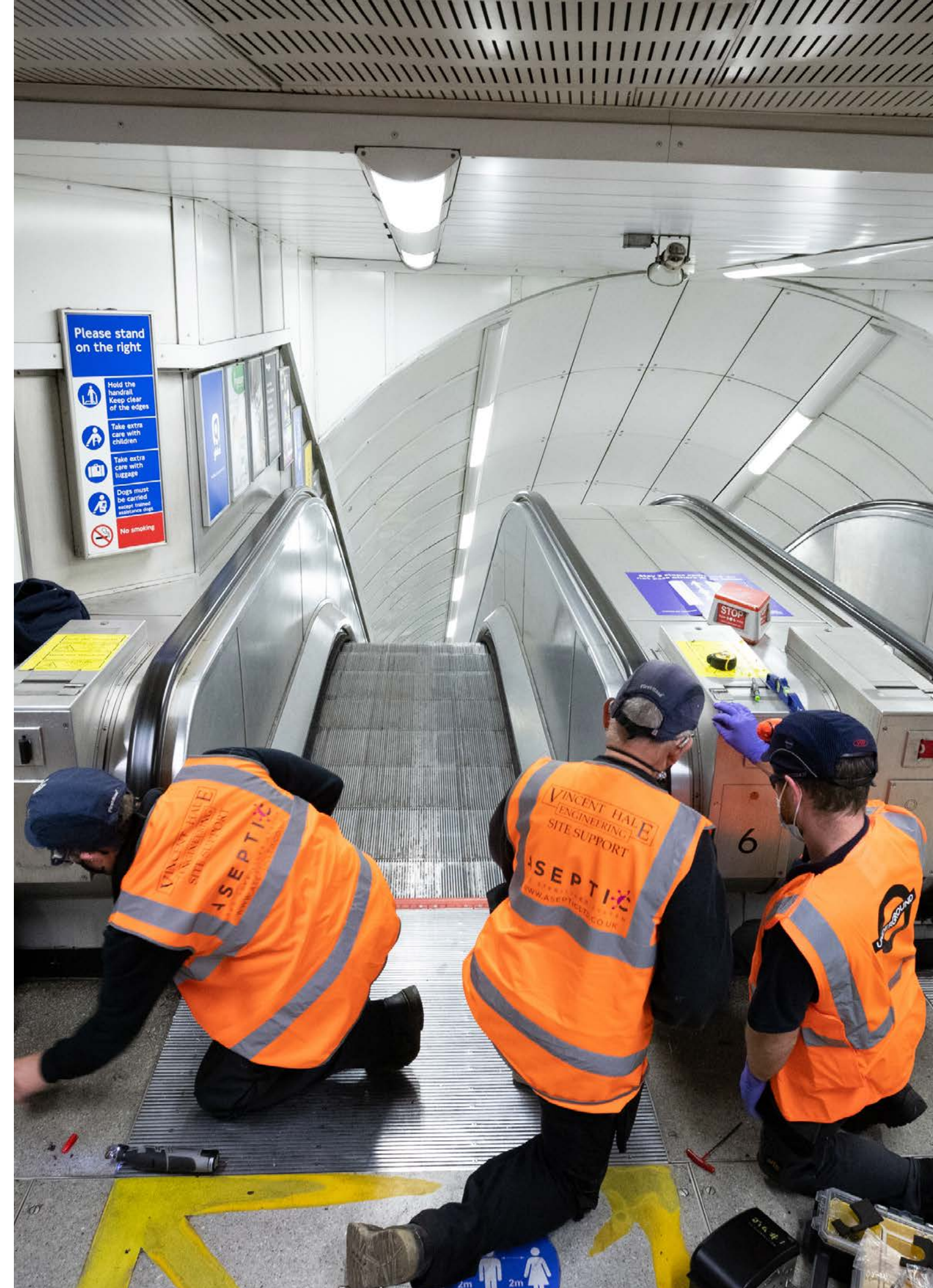
Our lifts and escalators need ongoing refurbishment and renewal
