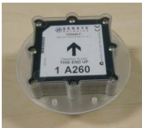
Magnetometer used as part of SCOOT installation
