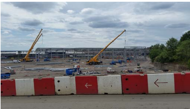
Construction of the Operations, Maintenance and Control centre at Old Oak Common
