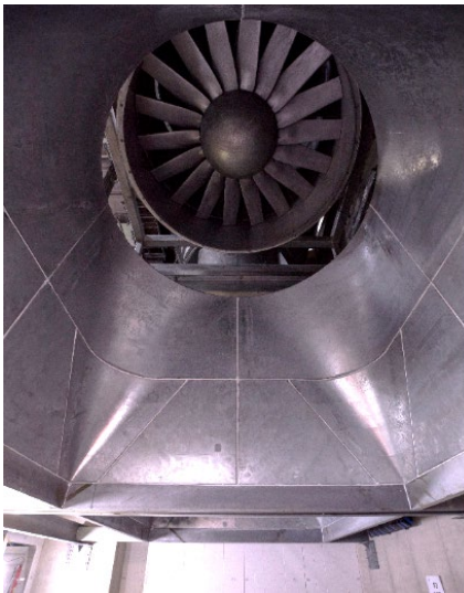
Figure 3 - Tunnel ventilation fan
