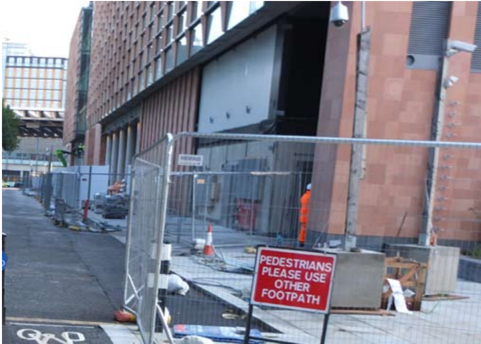
2 Brill Place is dominated by the bulk and massing of the Crick Institute.
