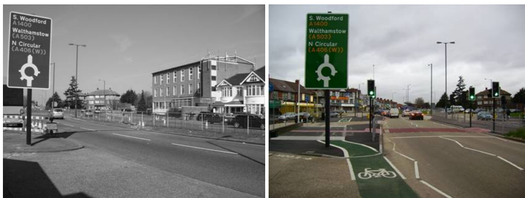
Figure 8.1 - Woodford Avenue before (left) and after (right) the implementation of the Toucan crossing
