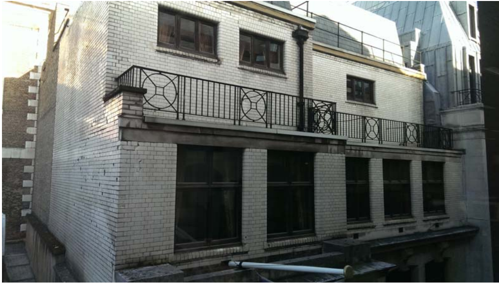
Photo 2: Damage to glazed brickwork on the upper levels of the Abchurch Lane façade
