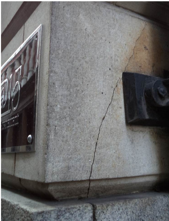
Photo 3: Detail of existing vertical cracks to the right hand side of the entrance foyer
