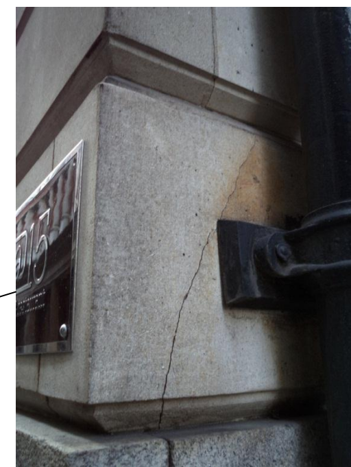
Areas of cracked stone and brick, and their location on the façade. Exact locations of the most vulnerable stone in need of repair to be verified by detailed condition survey
